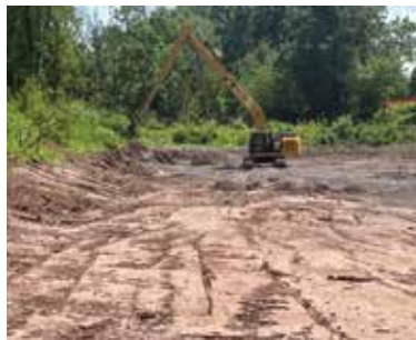
Work being done on the new bio-retention area at Enos B. Godshall Park
