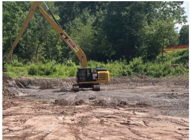
Work being done on the new bio-retention area at Enos B. Godshall Park
